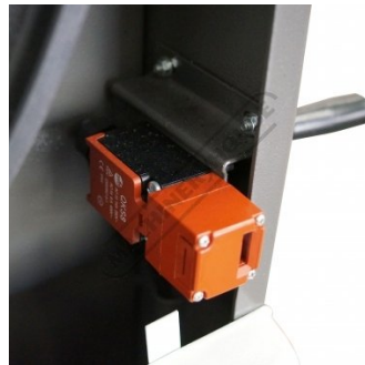
Safety Electrical Cut Out On Doors
