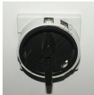
Main Isolation Switch
