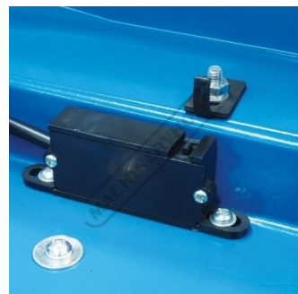
Safety Micro Switch on Pulley Guard
