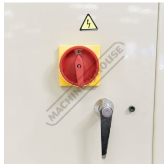
Main Isolation Switch
