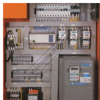
Electrical Control Cabinet
